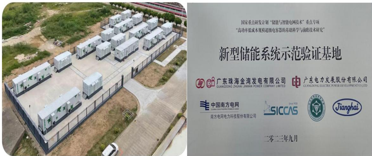
Figure 9-18 Energy Storage Demonstration Project in Zhuhai
