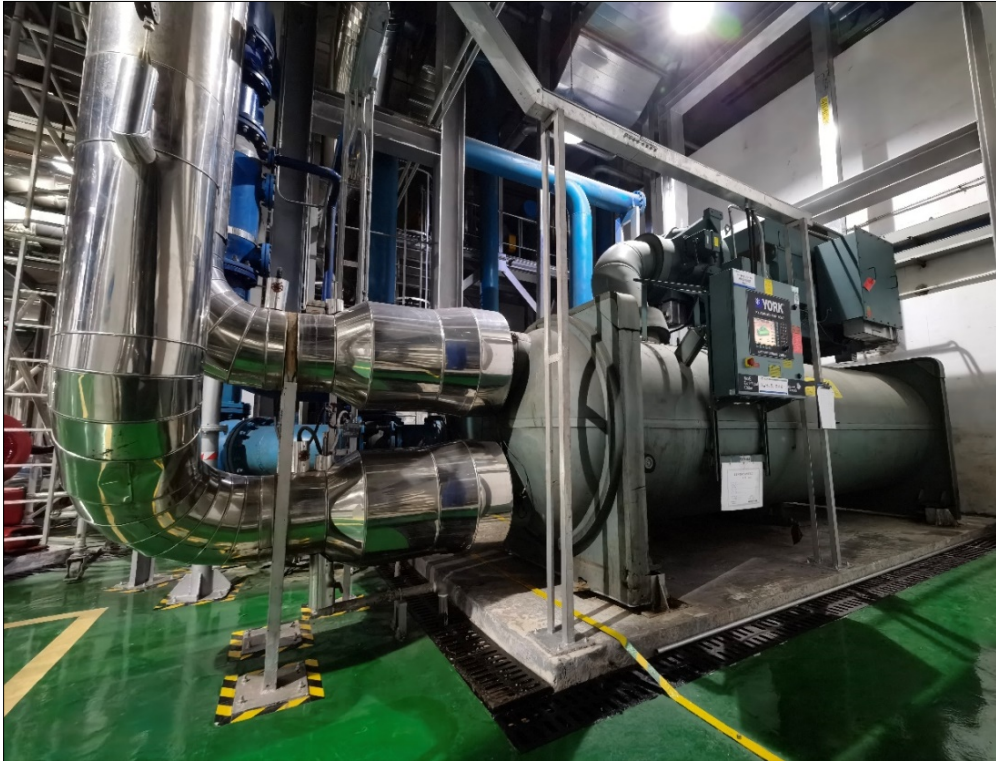
A base-load chiller unit for chilled water production for district cooling. Chilled water storage can directly be connected to the unit without extra retrofitting ( image courtesy of Jianping Fu, Shenzhen Qianhai Energy Technology Development Co., Ltd. ).
