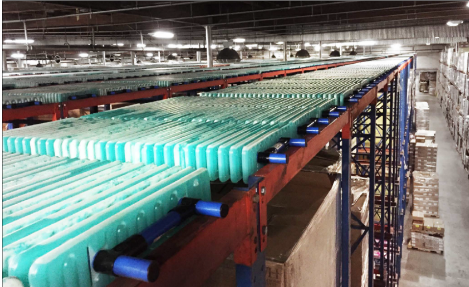
TES modules containing PCM installed above food storage racking (Viking Cold Solutions Inc. 2016).
