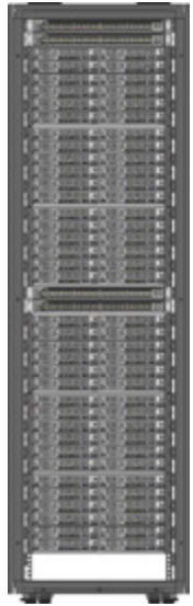
整机柜交付水冷单柜
