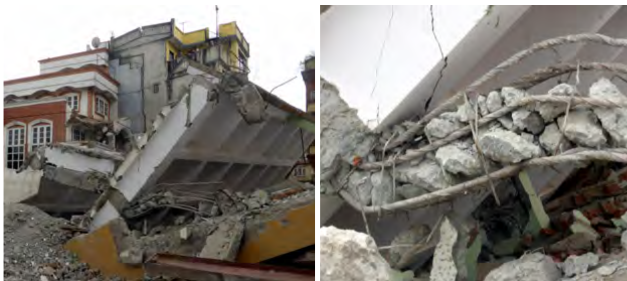
Figure 5.5 // The collapse of this reinforced concrete building in Kathmandu, Nepal during the 2015 Gorkha earthquake can be attributed to substandard quality of concrete construction, and a lack of ductile detailing of transverse reinforcement in reinforced concrete columns
