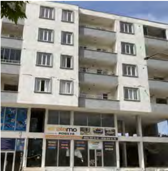
Figure 5.3 // Example of a reinforced concrete frame building with a soft story irregularity in the bottom two floors in Türkiye
