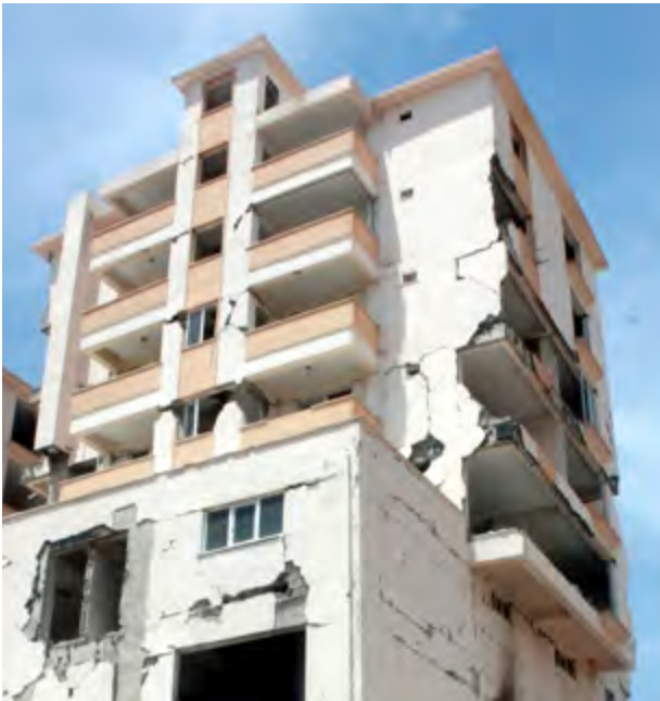
Figure 5.10 // Nonstructural URM exterior walls experienced damage or collapse in mid- and high-rise RC buildings due to the February 2023 Türkiye earthquake sequence, which can be attributed to inadequate connections between the intersecting walls and their anchorage to floor system
