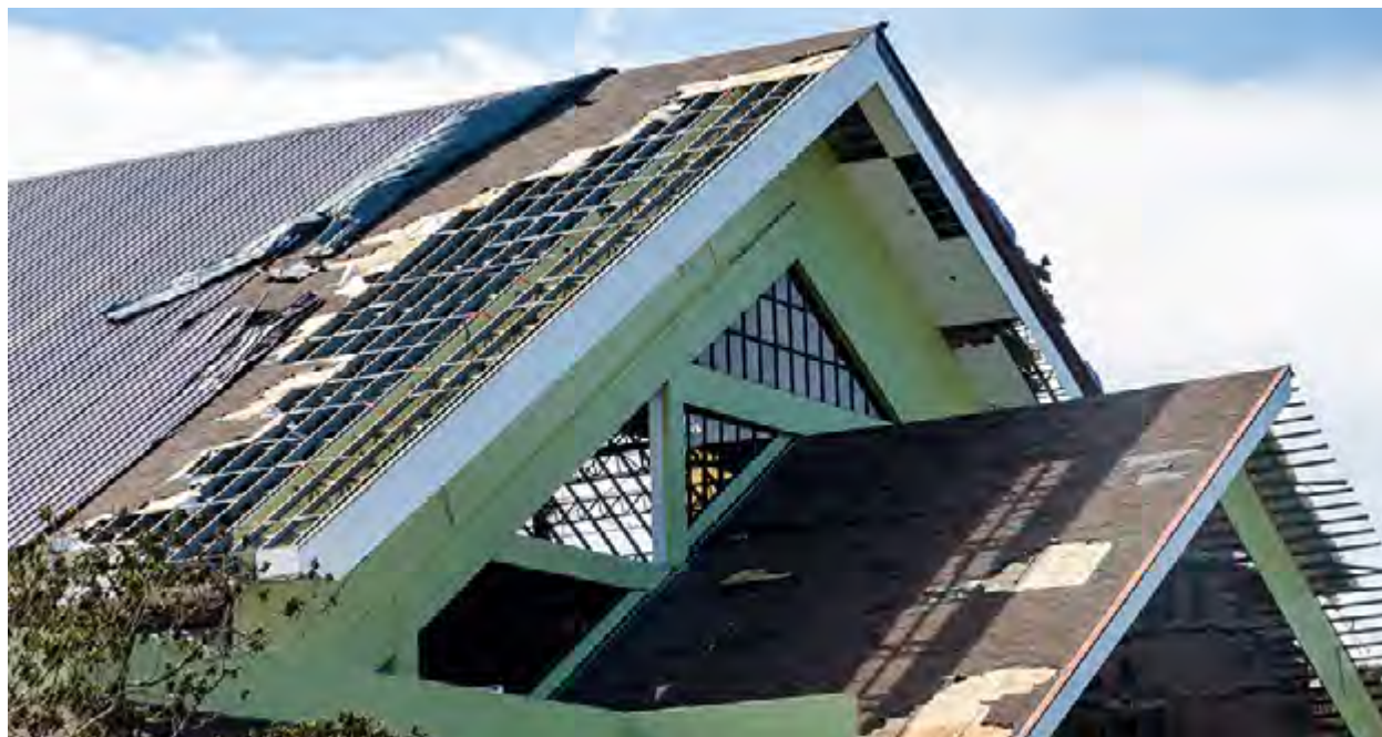
Roof damage from Super Typhoon Haiyan, Philippines. Photo credit: WhitcombeRD | iStock
