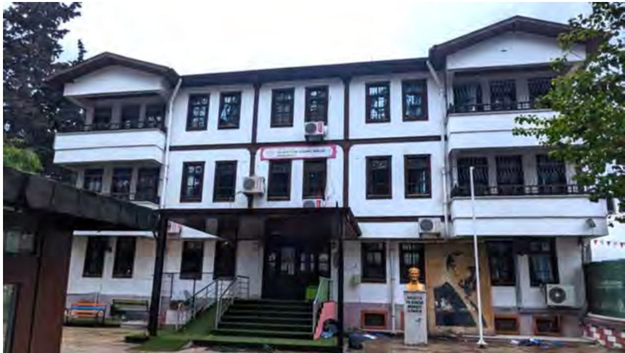
Figure 5.12 // School in Defne, Hatay, Türkiye, which experienced minor damage after the February 2023 Türkiye-Syria earthquake sequence
